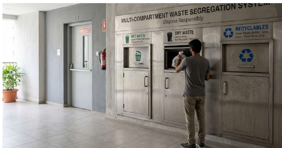
Figure 3: Multi-compartment Stainless Steel garbage chute system for Wet Waste, Dry Waste, and Recyclable Waste segregation
